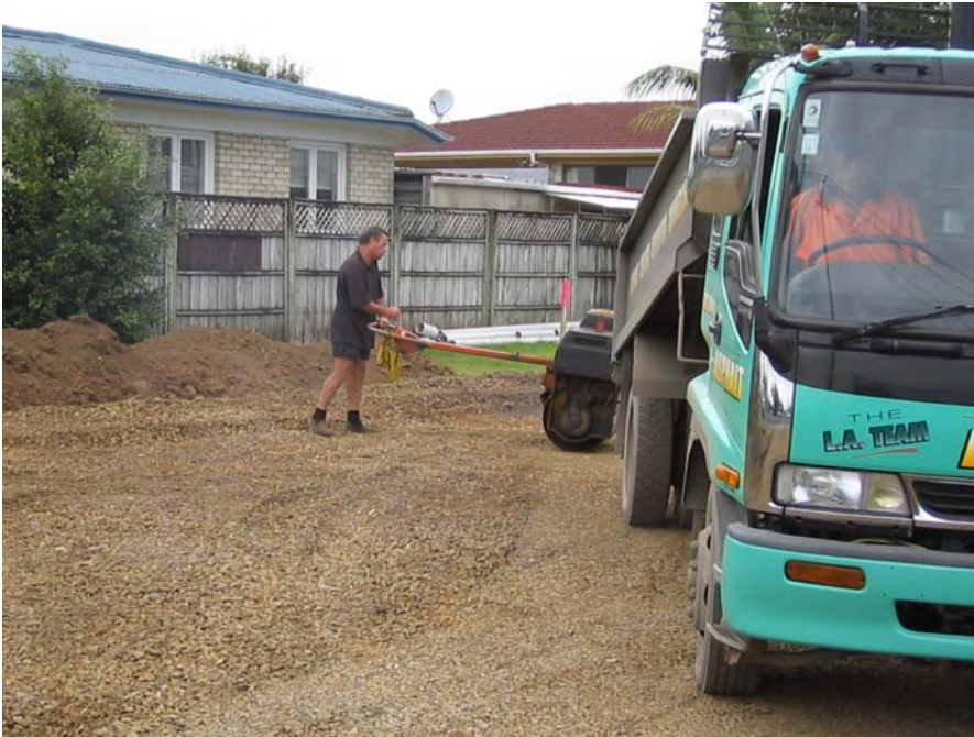
The parking area taking shape. Park here and stroll to the main entrance in Coronation Road.
